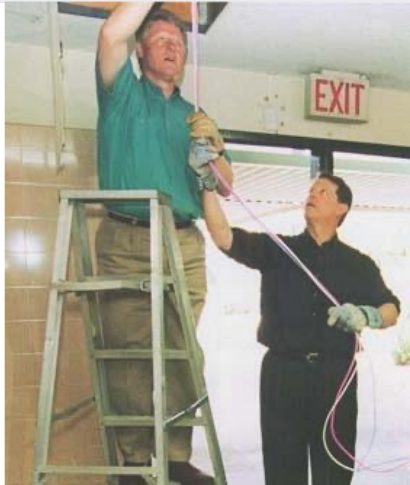
President Bill Clinton and Al Gore install computer cables on NetDay at Ygnacio Valley High School in Concord, California, 1996
