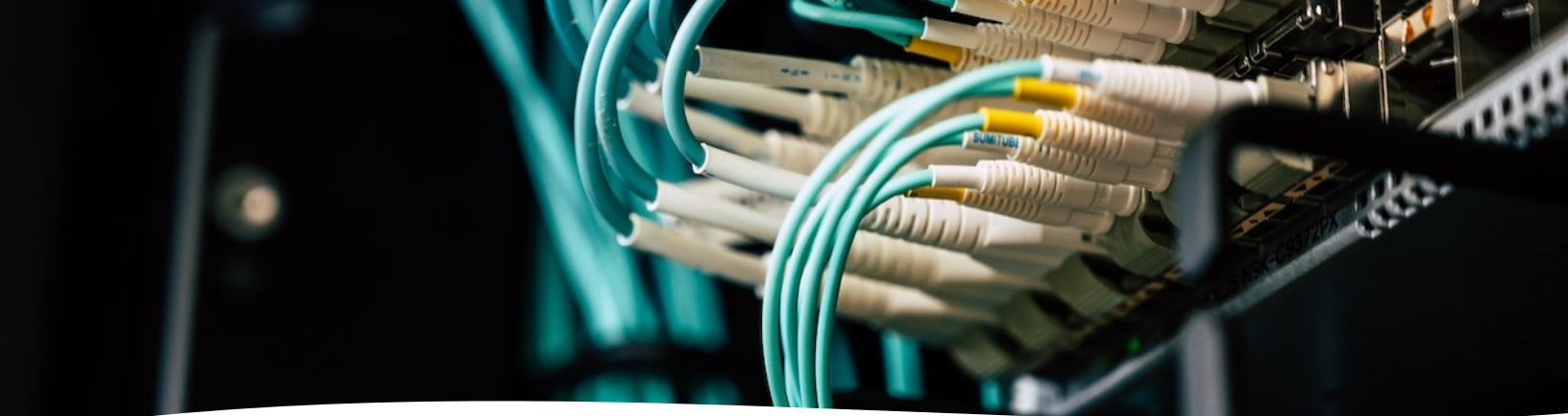
Cables connected to panel patch server
